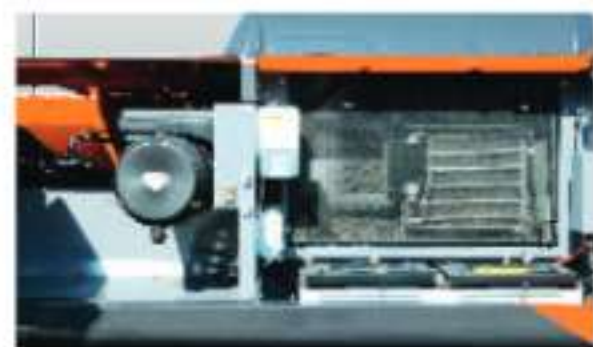
Utility space and radiators
