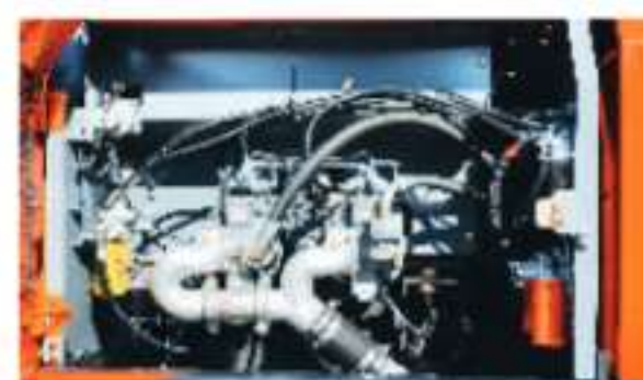
Grouped remote filters and inspection points
